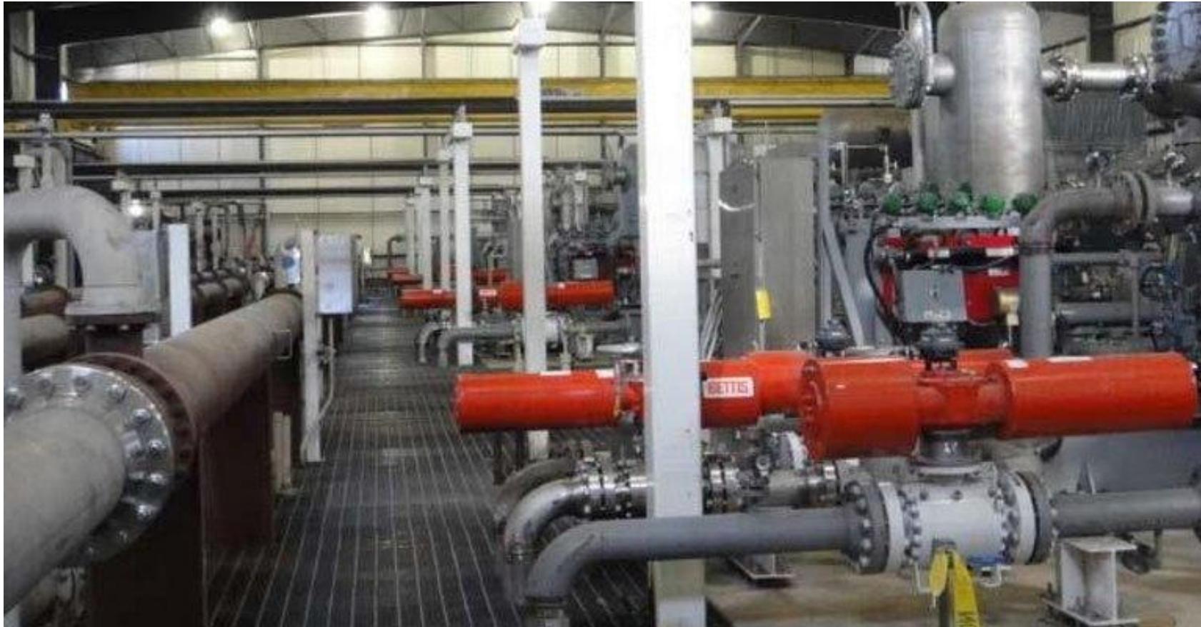
Inter-stage piping in the compressor facility (photo ADM) ADM CCS operation at Decatur, Ill ethanol production plant
